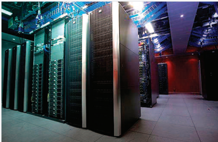
The Data Centre at the Sanger Institute.
